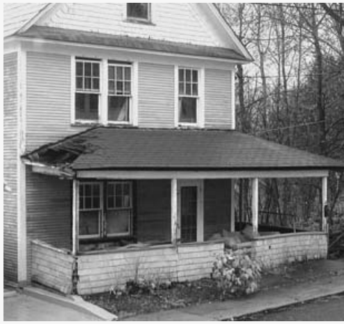
Disrepair is evident at this rental property in an Adirondacks town. Social workers say less visible interior problems are common, such as faulty wiring and malfunctioning heating systems.
