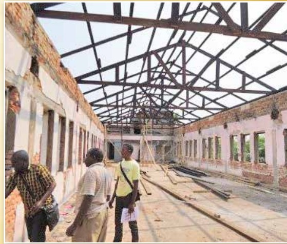
Spirits are going up along with the walls, as RSCJ in the Congo use the gifts from donors in the United States and Canada to rebuild dormitories destroyed by fire.
